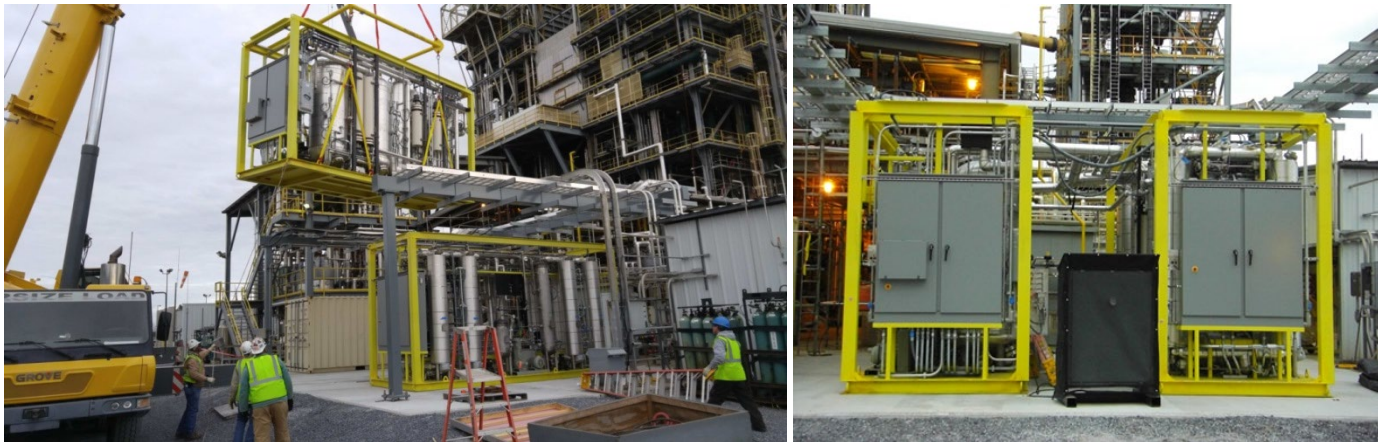
Figure 4: TDA's 0.1-MWe pilot unit installed in the test pad at the NCCC (Wilsonville, Alabama).
