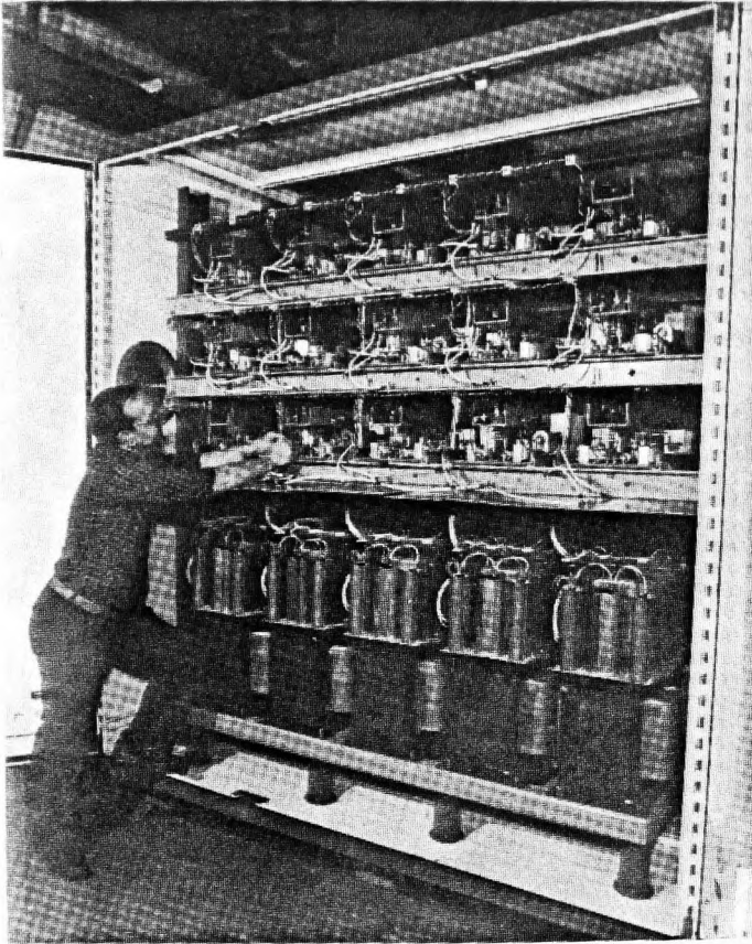
Figure 23. Anode Power Cabinet
