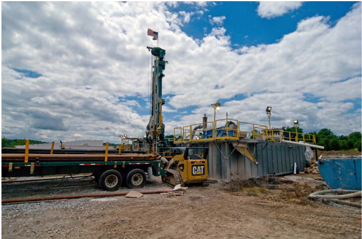
Figure 3-5. Photograph of Steel Tank Used to Contain Drilling Fluids and Drill Cuttings
