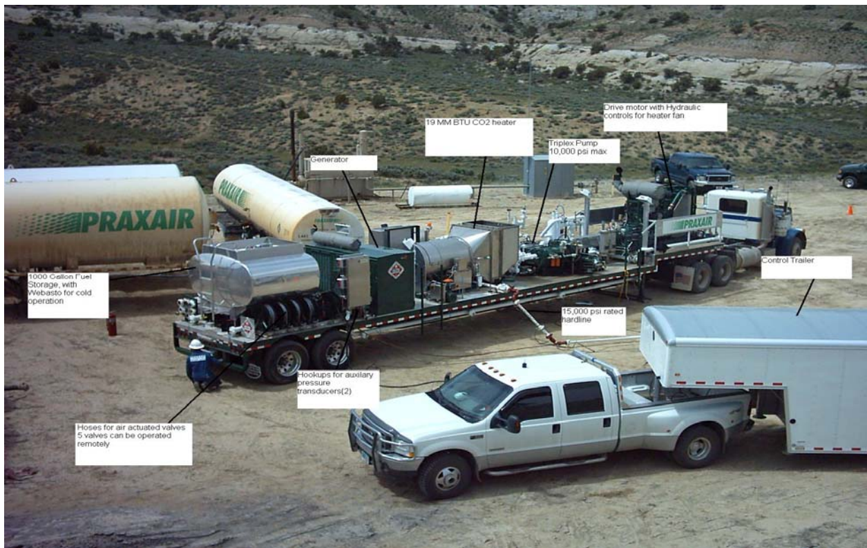
Figure 5-2. Equipment for CO 2 Injection Test
