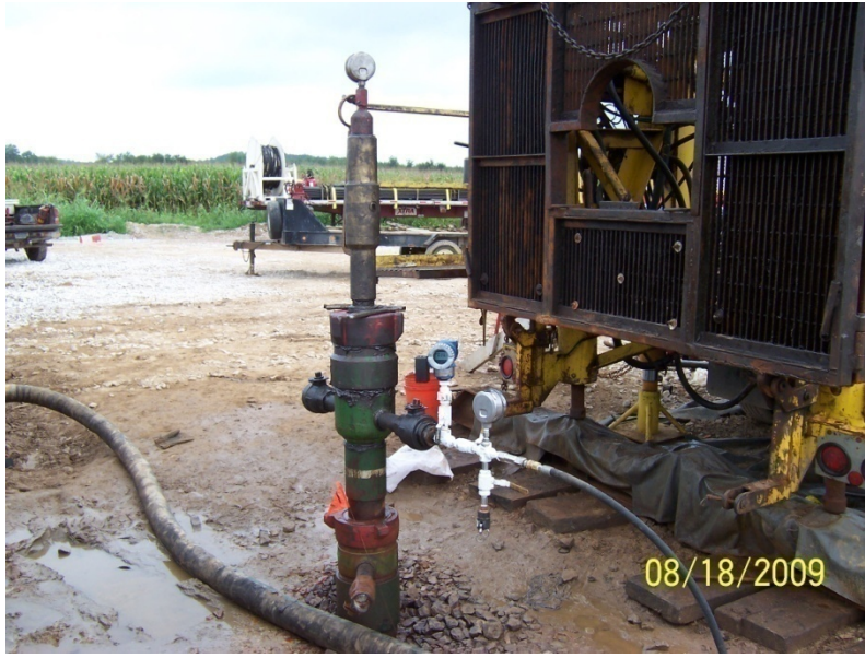
Figure 5-1. Conducting the Annular Pressure Test Prior to the Start of CO 2 Injection
